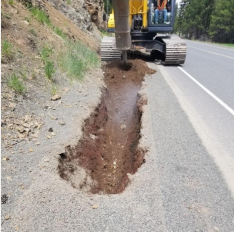
Photo 3: Excavating a trench using a rock hammer (photo credit: Zayo Group, LLC).
