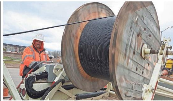
Jeff Jones, with ECL, a contractor for Midco, blows in fiber optic lines April 20 at the corner of 57th Street and Sycamore Avenue in Sioux Falls.
